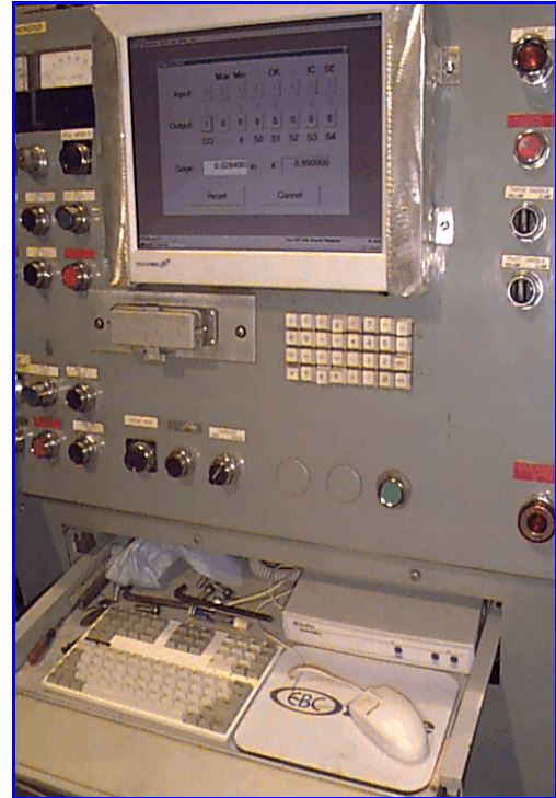
Figure 2. PC was placed inside an existing panel.
